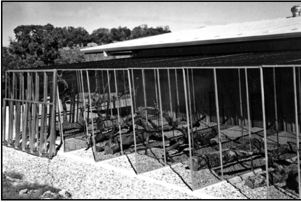
The outdoor cages as the wire panels were being assembled. Black PVC-coated, welded wire mesh was used. Each vertical panel sits on a 4-inch-wide concrete beam.
